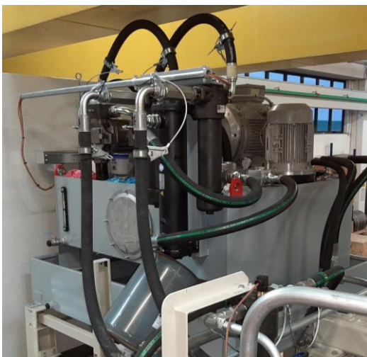
Hydraulic unit of the press for insulation panels
